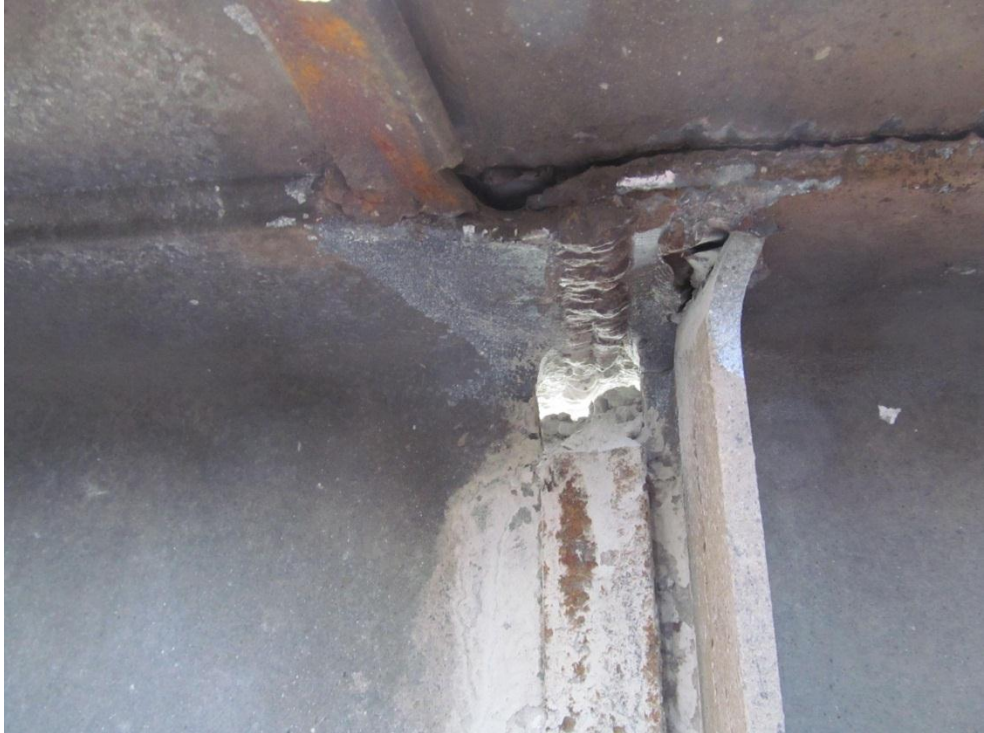
March 28, 2014 A3292 Pier 9 Expansion Joint Broken Strap
