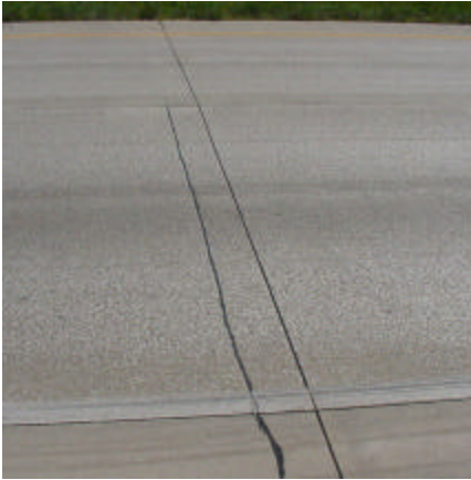
Figure 11. Crack at Mile Marker 94, RT 44
