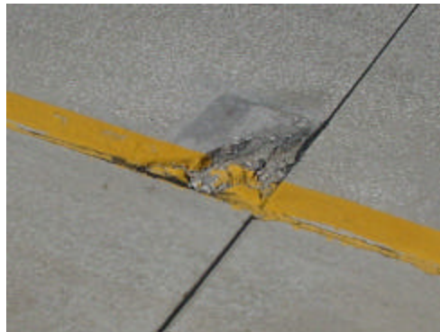
Figure 13. Damage at edge joint intersection at Station 72 + 00, RT 44
