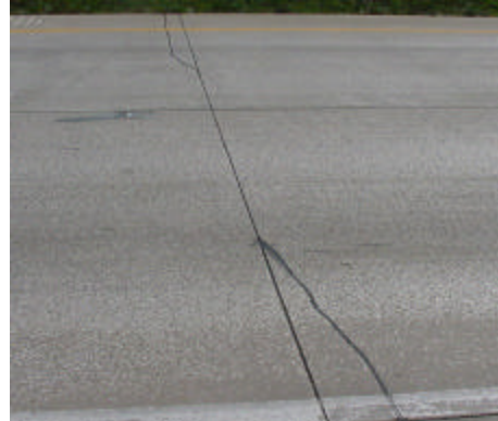
Figure 12. Cracks at Station 74 + 00, RT 44
