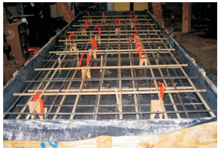
Fig. 1-The hybrid GFRP/CFRP (alternate bars) reinforced full-scale bridge deck slab is ready for placement of the FRC (0.5% Vf, 2" long fibrillated polypropylene fibers) matrix.
