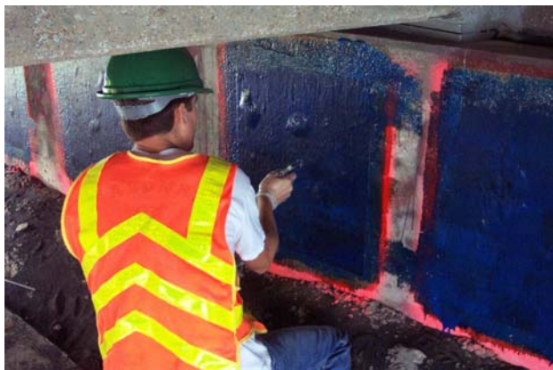
Figure 8 – Intentional defects in FRP laminates installed for evaluation purposes
