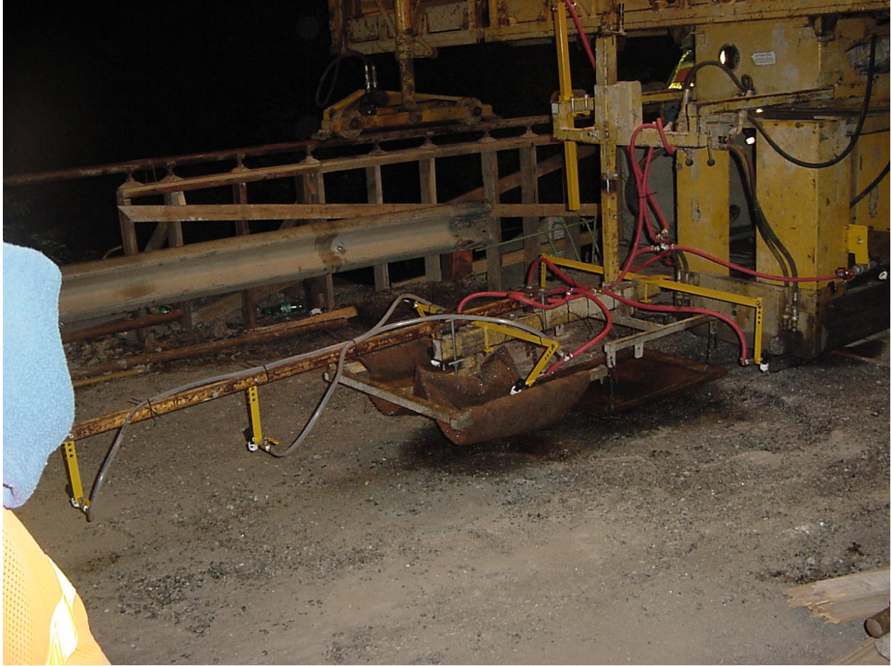
Figure 1: Close-up of fogging nozzles on pan screed, burlap drag and arm behind Bidwell finishing machine.
