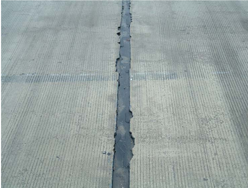
Figure 3: Edges broken off overlay on Bridge No. A3582 and approach pavement at sawed expansion joint.
