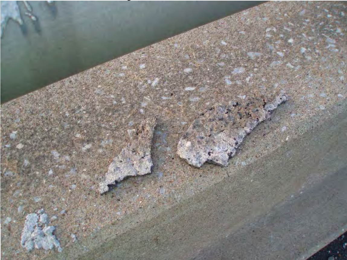
Figure 1. Epoxy Polymer Overlay that has concrete paste attached to the bottom
