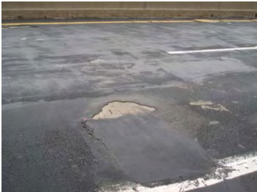
Missing areas of epoxy
