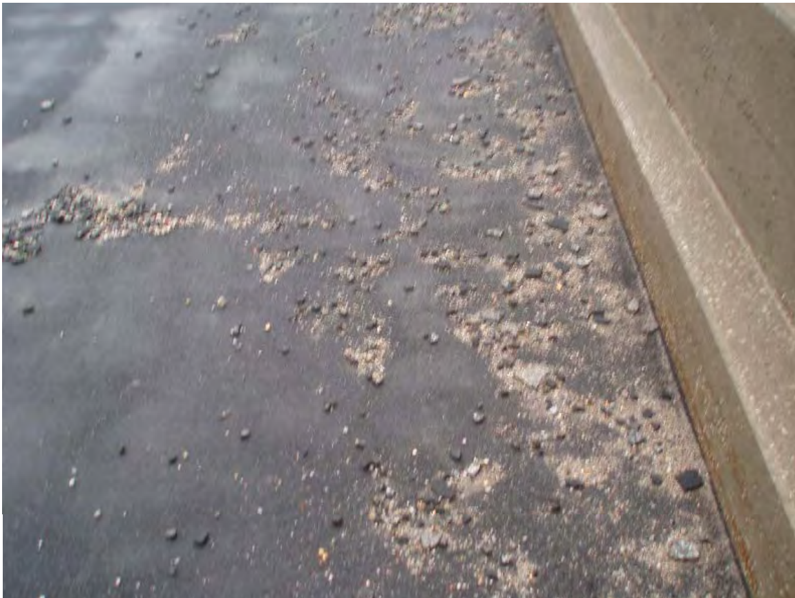
Figure 2. Epoxy “flaking” off the bridge deck
