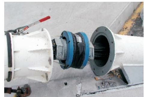
Figure 2: Damper at cable anchorage.
